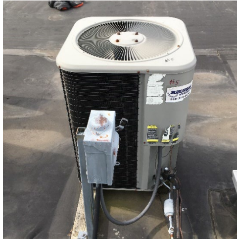
Rooftop Condenser (System #5)
