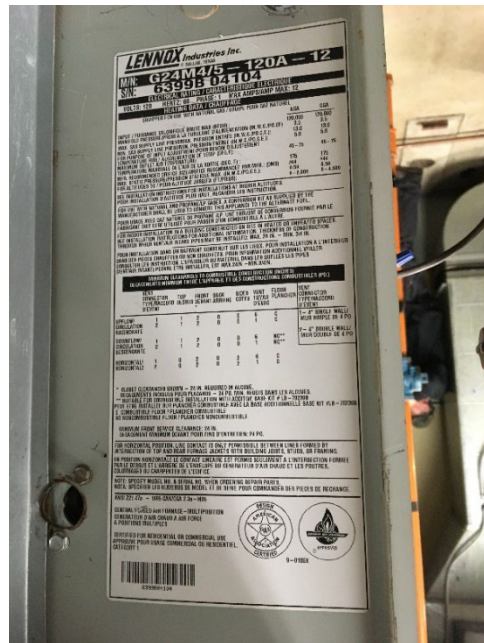
Furnace Faceplate (System #6)
