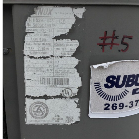
Condenser Faceplate (System #5)
