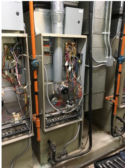
Gas Furnace (System #4)
