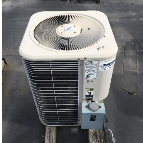
Rooftop Condenser (System #4)
