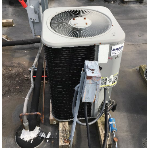
Rooftop Condenser (System #6)
