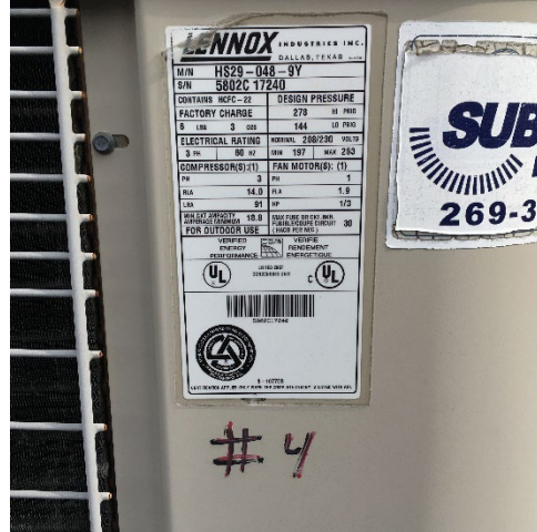
Condenser Faceplate (System #4)
