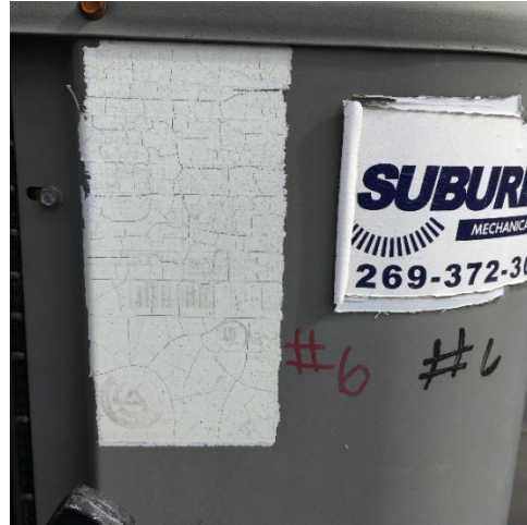
Condenser Faceplate (System #6)
