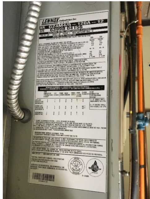
Furnace Faceplate (System #4)
